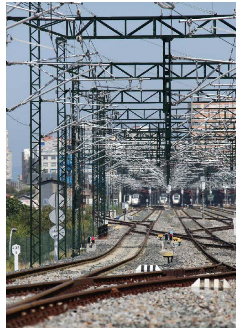
Catenary for the Atlantic Axis for ADIF (Spain).
