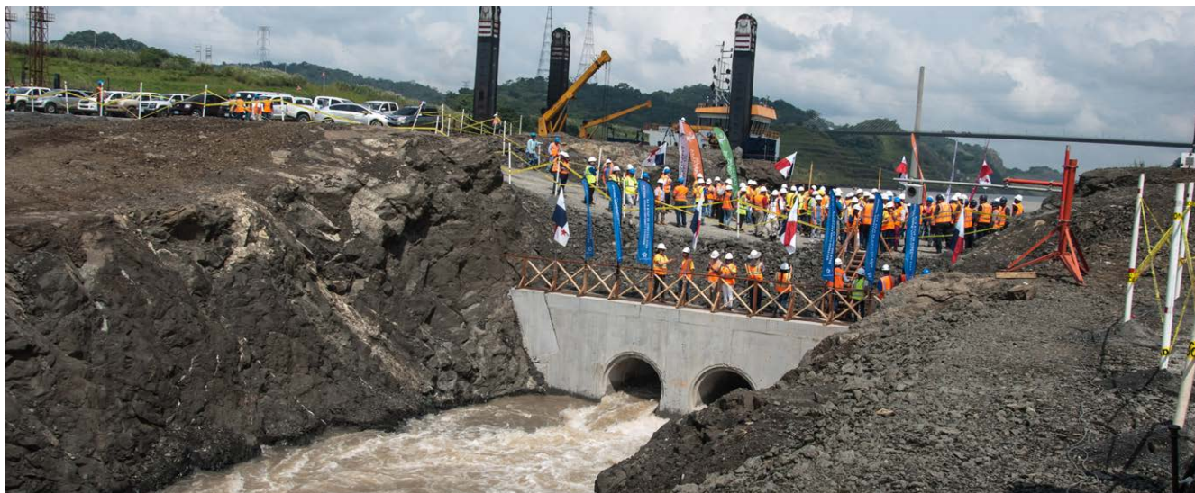
Filling tests of the PAC 4 in the Panama Canal expansion programme (Panama).
