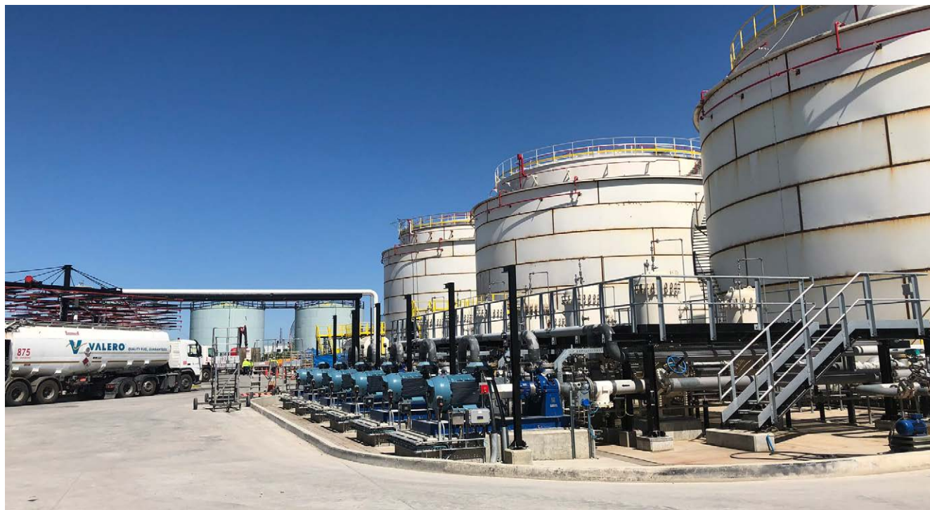
Fuel storage facilities at Dublin Airport, Ireland.
