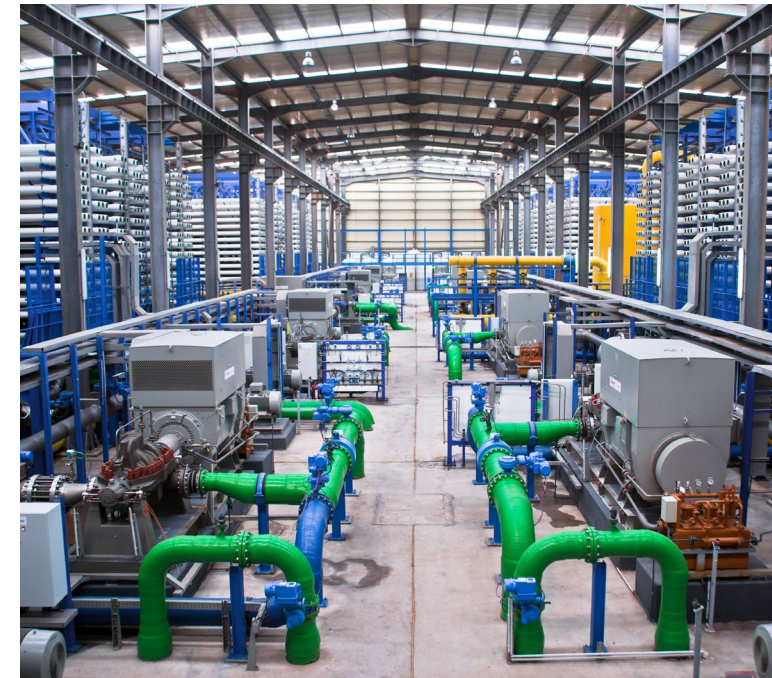
SWDP in Mostaganem (Algeria).
