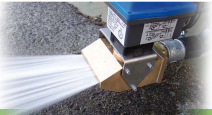
Installation of adjustable sluicing units with programmable automaton in the flushers.
