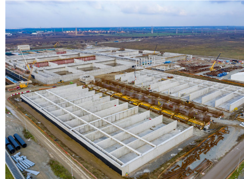
Wastewater treatment plant in Glina (Romania).
