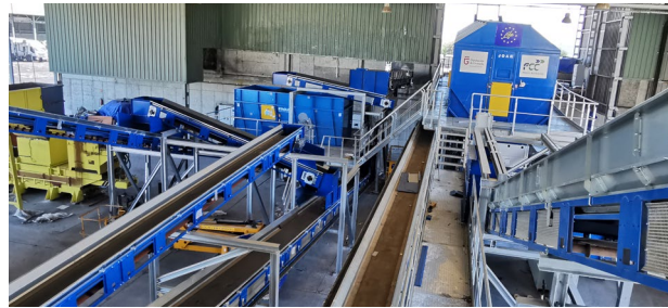
Life4Film treatment line in the Ecocentral plant, in Granada (Spain).
