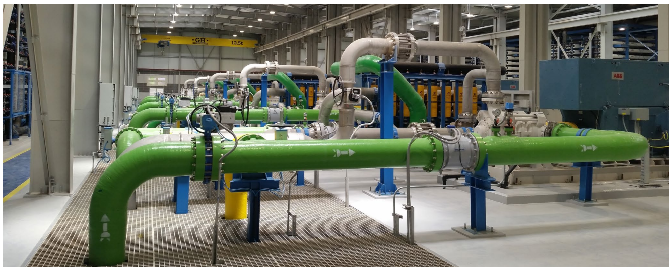
The El Alamein plant (Egypt), chosen as one of the three desalination plants of the year at the Global Water Awards.
