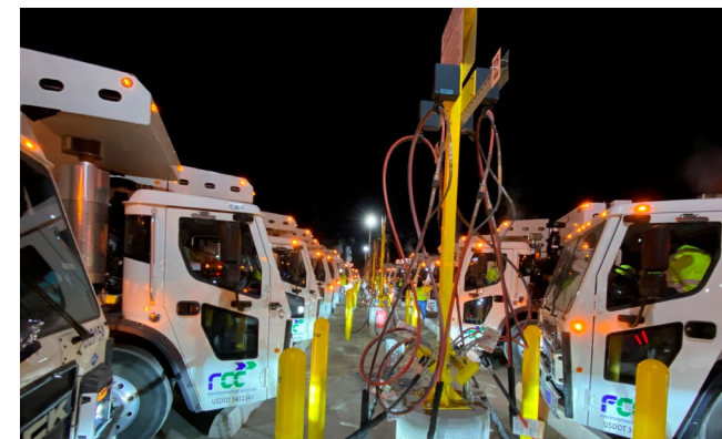
CNG Station Omaha, Nebraska (USA).
