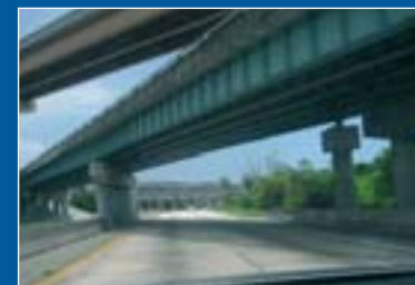
Detail of the two curved overpasses and third-level viaducts at the SR-112 intersection, on the right.
