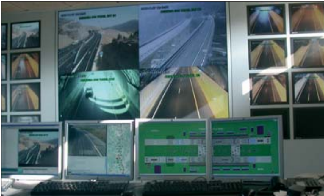
Above these lines, the interior of the Puig Reig-Berga (Barcelona) tunnel control center. On the right, the entrance of the Lomas de Bas (Cartagena) tunnel.
