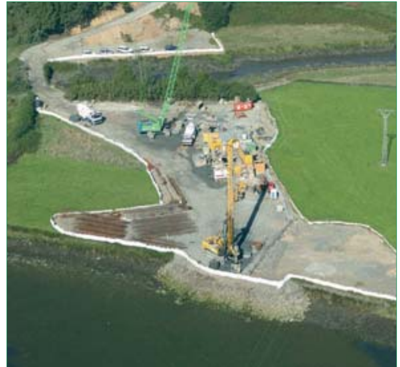
Fencing in the work site improves security and reduces as much as possible the affected area during the execution of a project.
