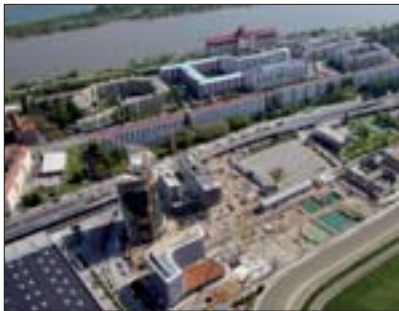
The hotel's sweeping form curves towards the neighboring Hoch Zwei building, which Alpine is also building.
